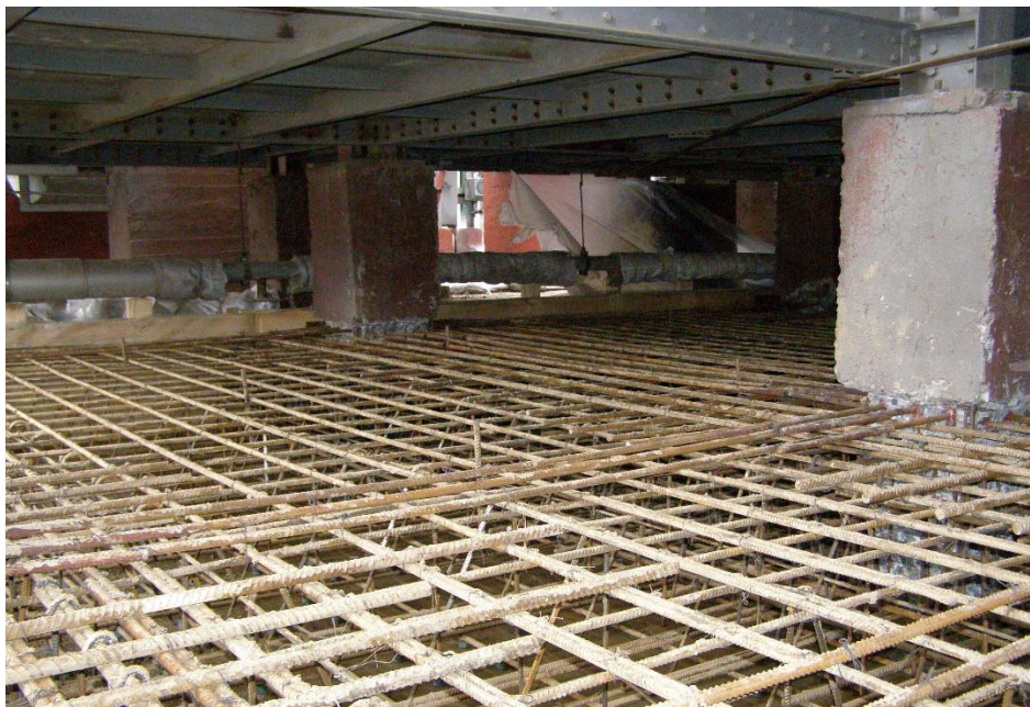
Figure 1 – The stage of installation of reinforcing frames of the slab of reinforcement of the foundations of the furnace
